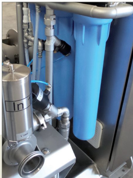
Washing water filtration
